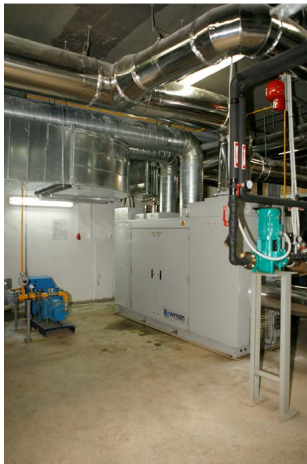
Fig.2 : View of the installation
