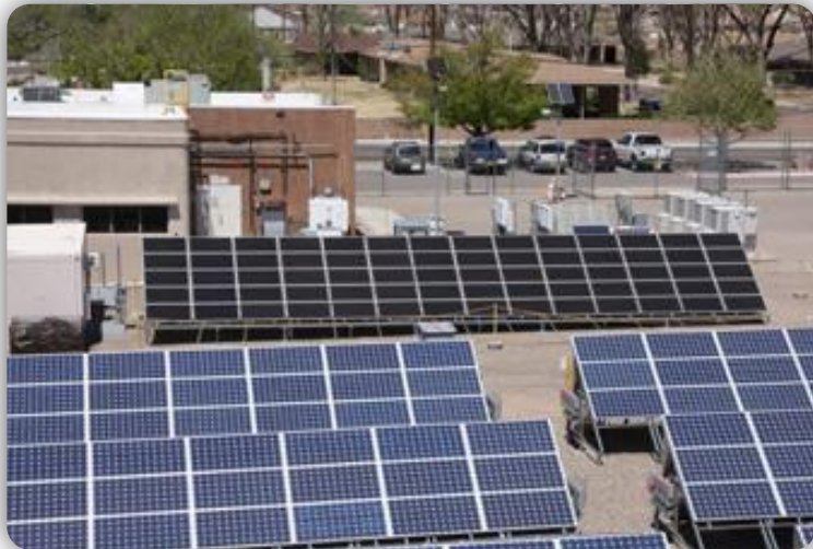
High penetration PV Systems at SANDIA DETL
