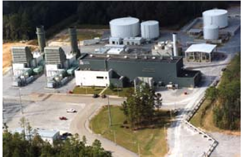
Compressed Air Electrical Storage
